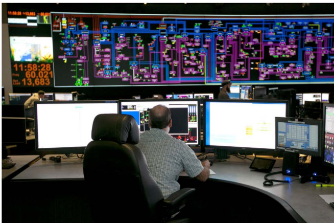
A grid control center for Pacific Gas & Electric, a major California utility. Power companies, particularly in the West, are accelerating their shift from natural gas to renewable sources. Rob Pedroncelli/Associated Press
